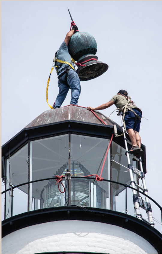
John Xipolitus and Anthony Presutti of Razorback LLC reinstall the repaired vent ball.
